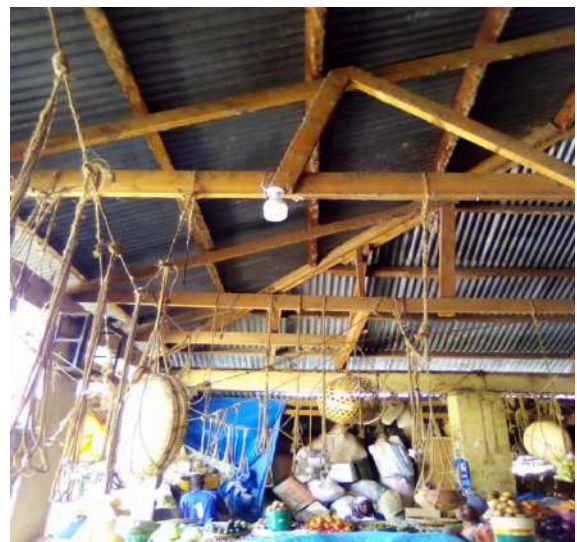
Photo 5: Soko Kuu market in Mara Region with installed electricity. (Source, EfG, 2021)
